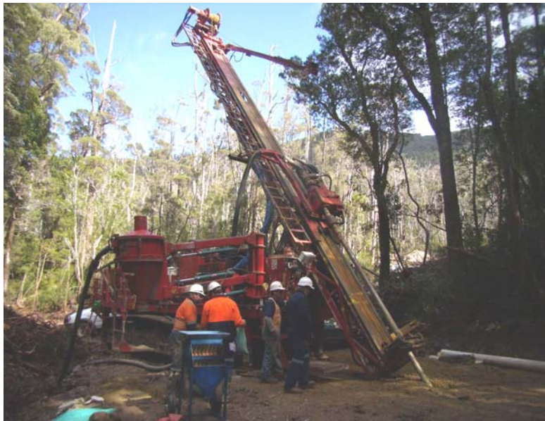
Multipurpose Drill Rig drilling the first Reverse Circulation drill hole at Stanley River
